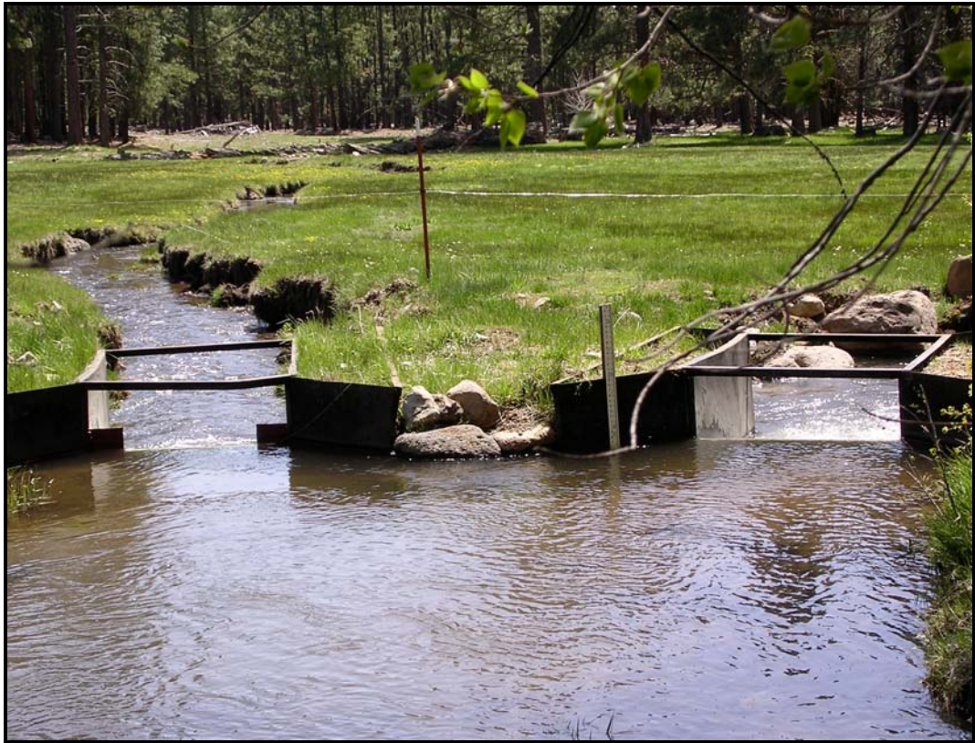
Photo 8-1. View of Diversion and Unstable, Eroding Banks on Jackson Creek
