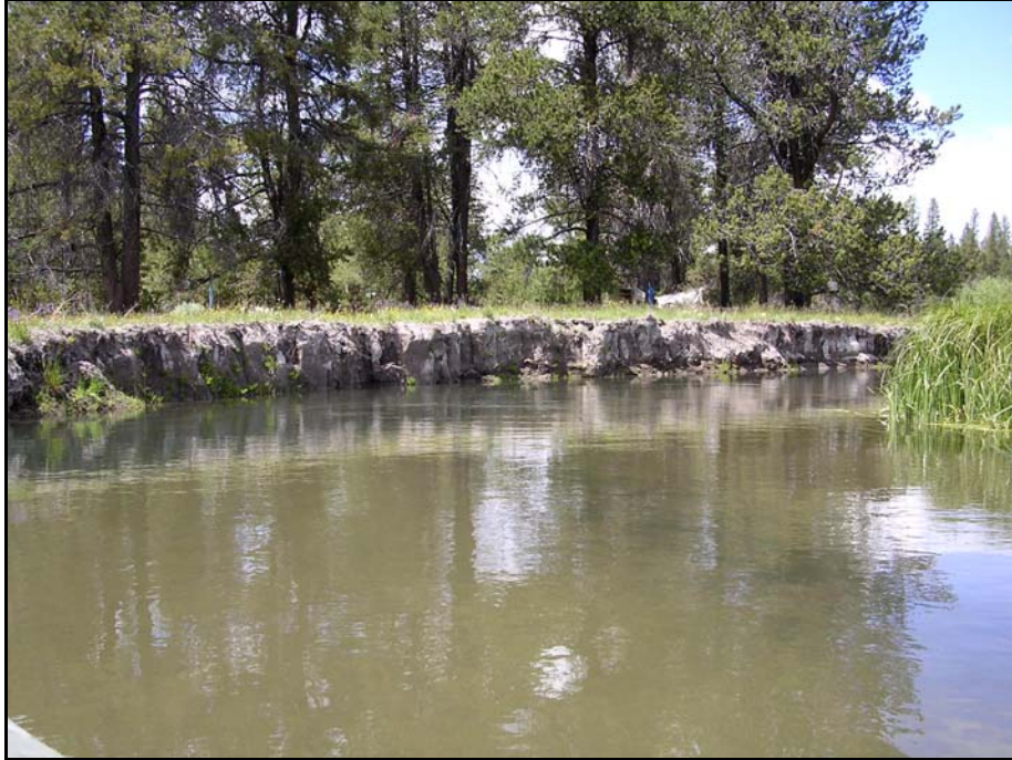
Photo 8-4. View of Typical Bank Erosion between Deep Creek and Rocky Ford
